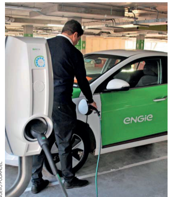
Santiago airport parking lots are equipped with electric chargers to encourage electric mobility.
